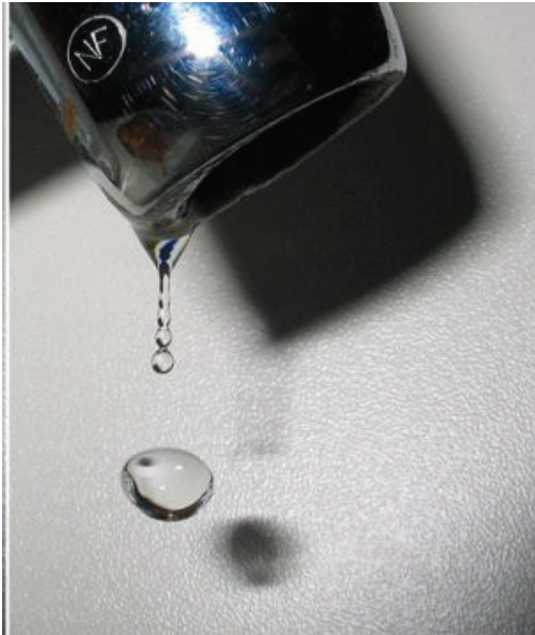
Figure 18.18: One drop per second from a dripping faucet wastes 2,700 gallons of water per year and adds to sewer and/or septic costs, as well. (27)
